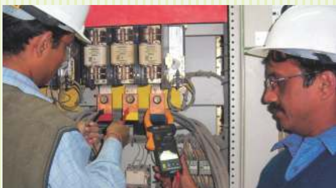
Measurement of Electrical Parameters with Clamp-on Power Meter
