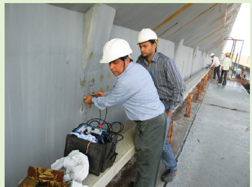
Measurement of crack depth using UPV technique on sea side RCC basin wall of cooling tower unit III of Dabhol Power Project, Ratnagiri
