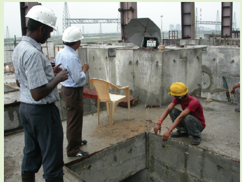
UPV testing being carried out on cross beam of Turbo Generator Deck at NTPC Barh, Patna
