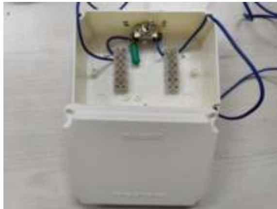
Monitoring junction box assembled for periodic monitoring of performance of anodes
