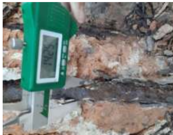
Measurement of existing rebar diameter of an RCC member at a Building site in Delhi
