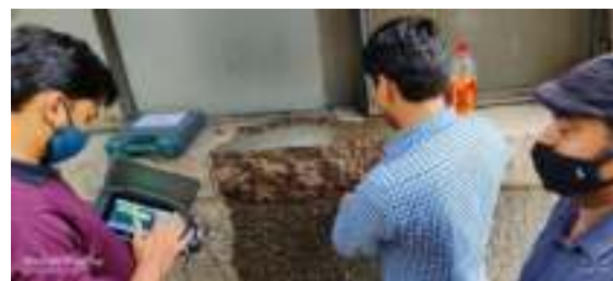
Measurement of Half-Cell Potentials of reinforcement on an identified beam in NCB premises
