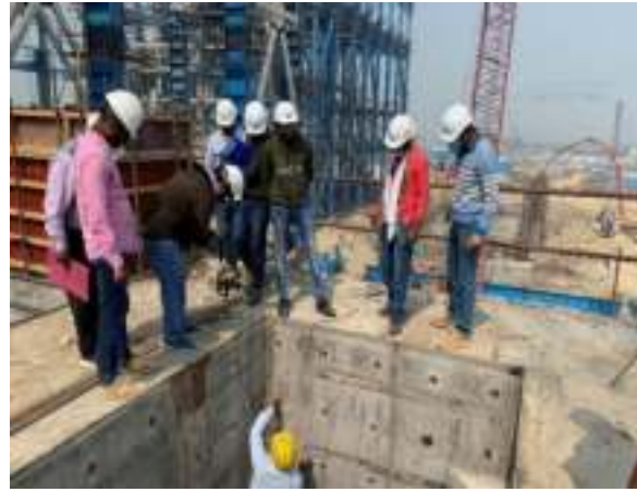
UPV Test on TG Deck Slab at a power plant project site in Uttar Pradesh
