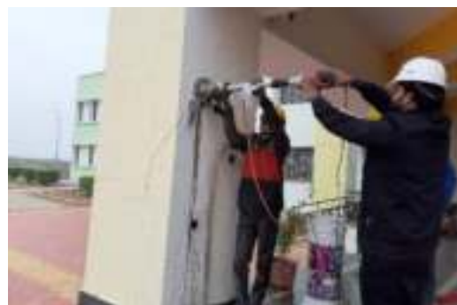
Concrete Core Extraction from RCC Column of Township Building at NTPC Gadawara
