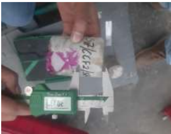
Carbonation depth being measured on freshly extracted concrete core at a Hospital Building site
