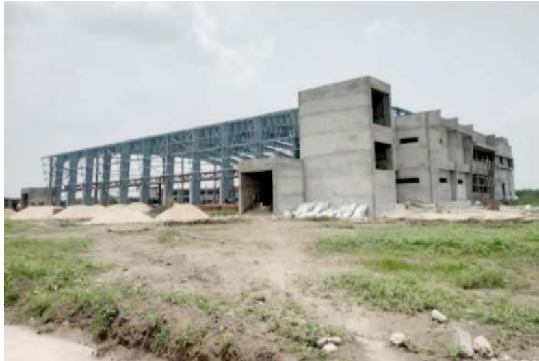
Multipurpose Hall at Desar A glimpse of Third Party Inspection & Quality Assurance project at NCB-Ahmedabad
