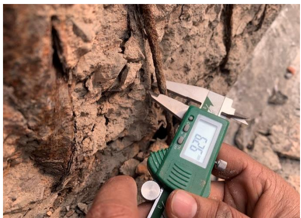
Measurement of existing rebar diameter as part of site investigation for a corrosion damaged structure
