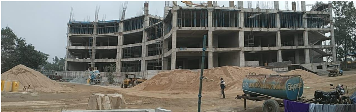
IDCO Tower, Jharsuguda
