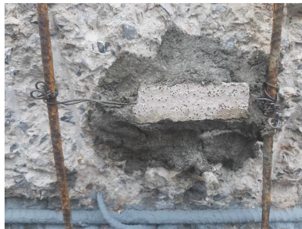
Installation of sacrificial anode at site for field study under R&D project on Cathodic Protection of Reinforced Concrete
