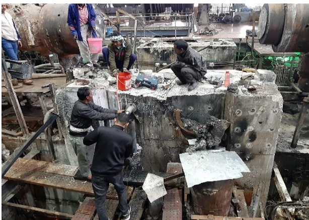
Site Investigation on Fire damaged TG Deck
