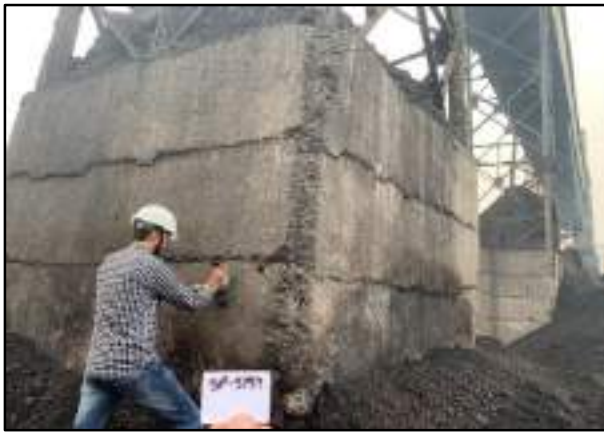
Ferro scanning test on RCC pedestal of Conveyer belt in Coal Handling Plant
