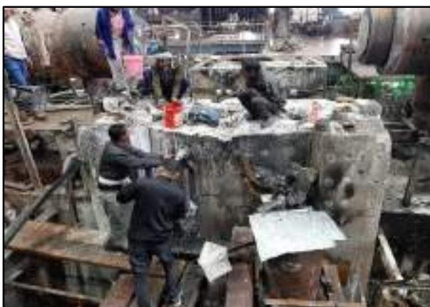
Site Investigation on Fire damaged TG Deck
