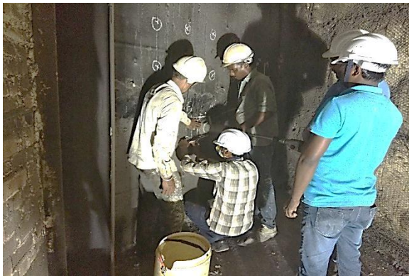
Extraction of Concrete Core from the Inner Shell of RCC Chimney of NTPC Ramagundam
