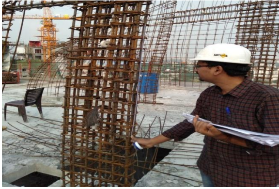
Checking of Lap length provided to a Column at IIT Madras campus
