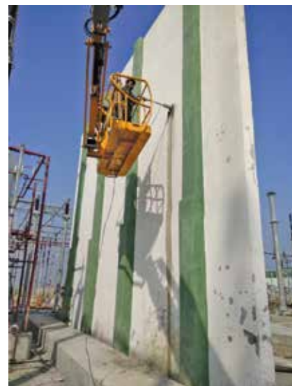
Extraction of Concrete Cores by NCB Team on Fire wall in 400KV Sub Station, Orai
