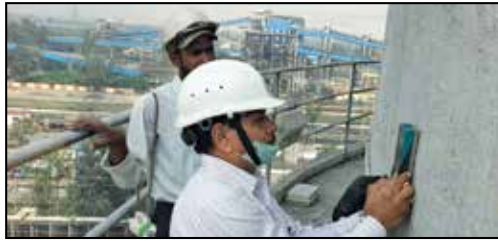
Profoscope Test in progress at 70M Elevation of Chimney at NTPC, Vindhyachal
