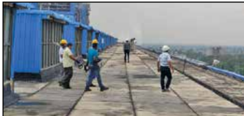
Inspection of TG Roof Slab Top by NCB team at NTPC Sipat
