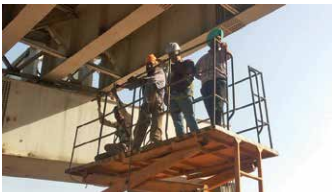
Inspection of HSFSG Bolts after Slab Concreting at PWD Flyover Project at Viaspuri, Delhi
