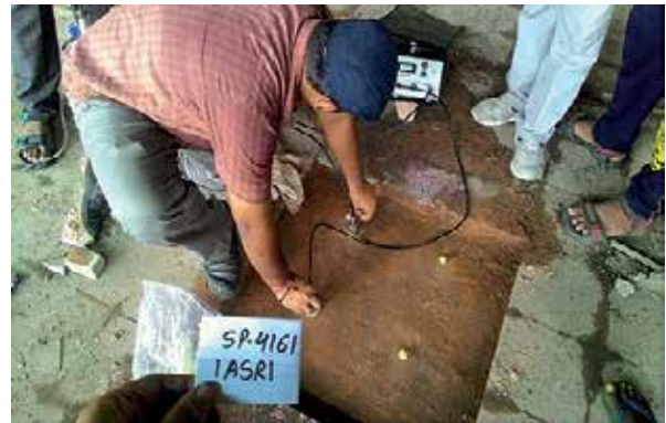
UPV Testing being done by Surface Probing on RCC Slab in the Sample Survey Block (Back Wing) at IASRI, Pusa, New Delhi
