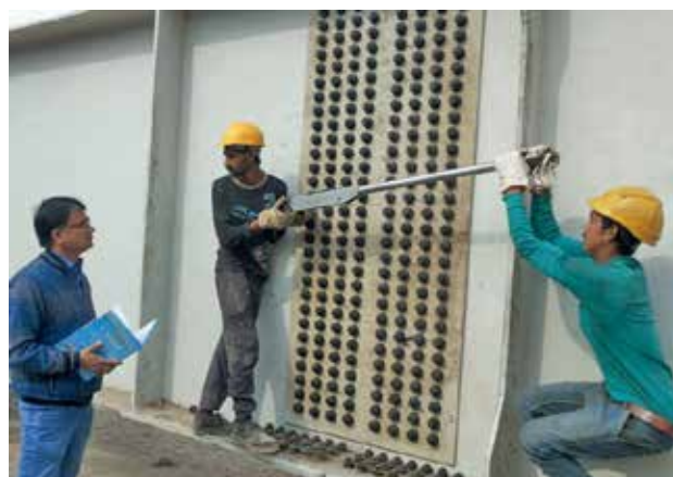
Checking of Torque of HSFSG Bolts at PWD Flyover Project at Viaspuri, Delhi
