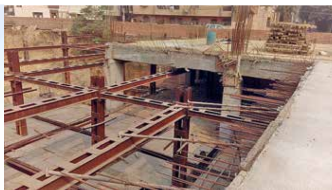
Underground Multilevel Car Parking of SDMC at Subhash Nagar, New Delhi
