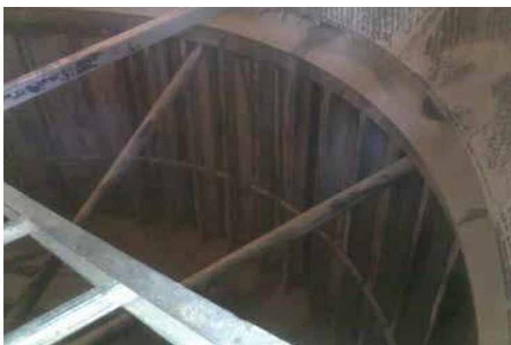
View of mill worn-out rotor and stator of the classifier of VRM
