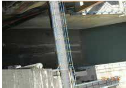
Erosion of concrete due to high velocity flow of water in the spillway of Nathpa Dam, HP
