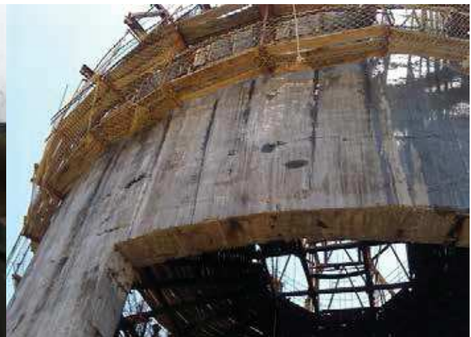
Apparently un-distressed outer face of chimney stack of BRBCL Aurangabad
