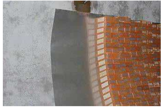
Use of sacrificing layer protects kiln shell from corrosion
