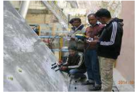
Pull off testing being carried out on the dam body of Nathpa Dam of SJVNL, Nathpa (HP)
