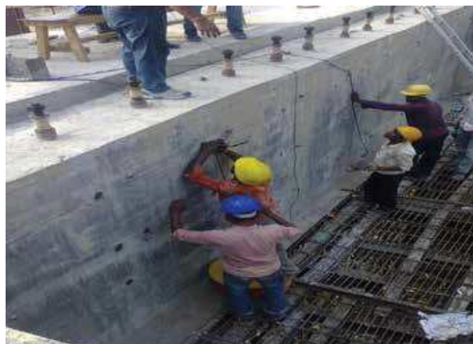
Measurement of UPV on longitudinal beam of TG deck Slab at NTPC-Lara
