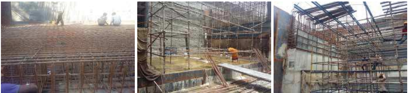
Third party quality assurance for construction of 2 nos RCC box underpass for PWD, Delhi
