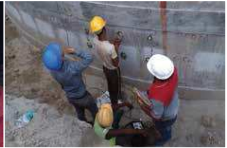
UPV Testing being done on RCC Wall of Well at Sewage Treatment Plant
