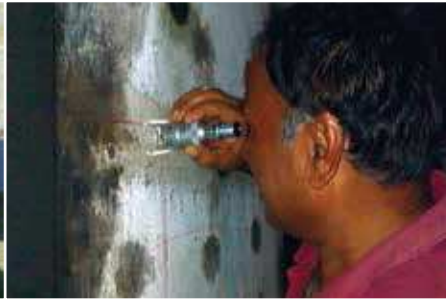
Crack width being assessed on RCC Column of TG Foundation by using Crackoscope
