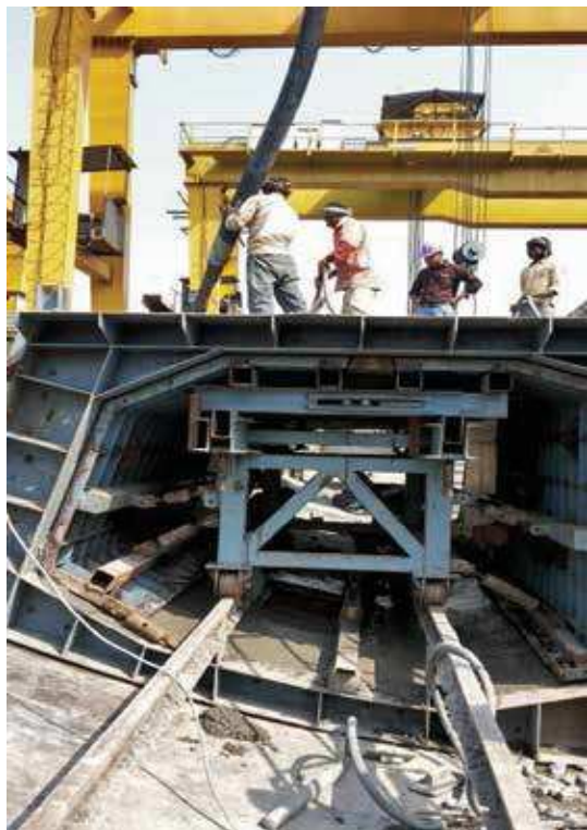
Inspection of Concreting of Pre-cast Spine Segment of Flyover Project at Viaspuri, Delhi
