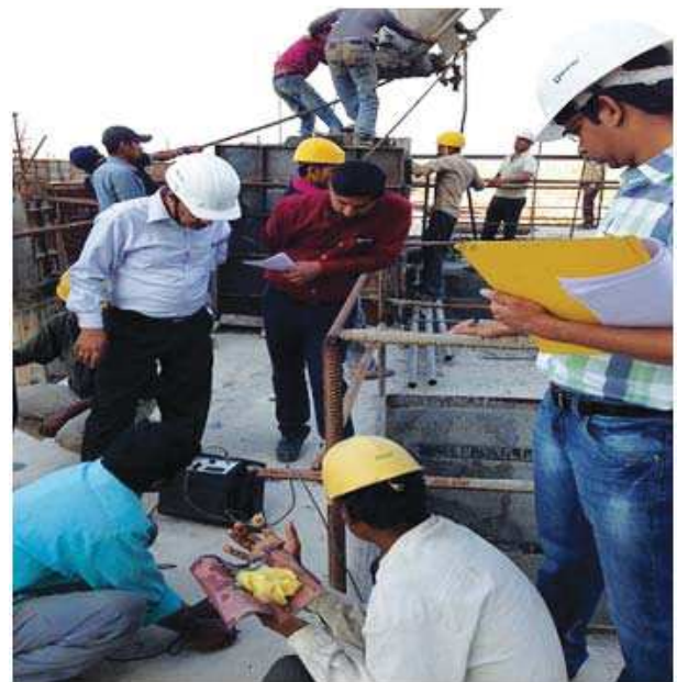
UPV testing being done on a TG Deck Slab for a Thermal Power Project
